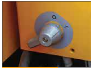
BATTERY DISCONNECT SWITCH
